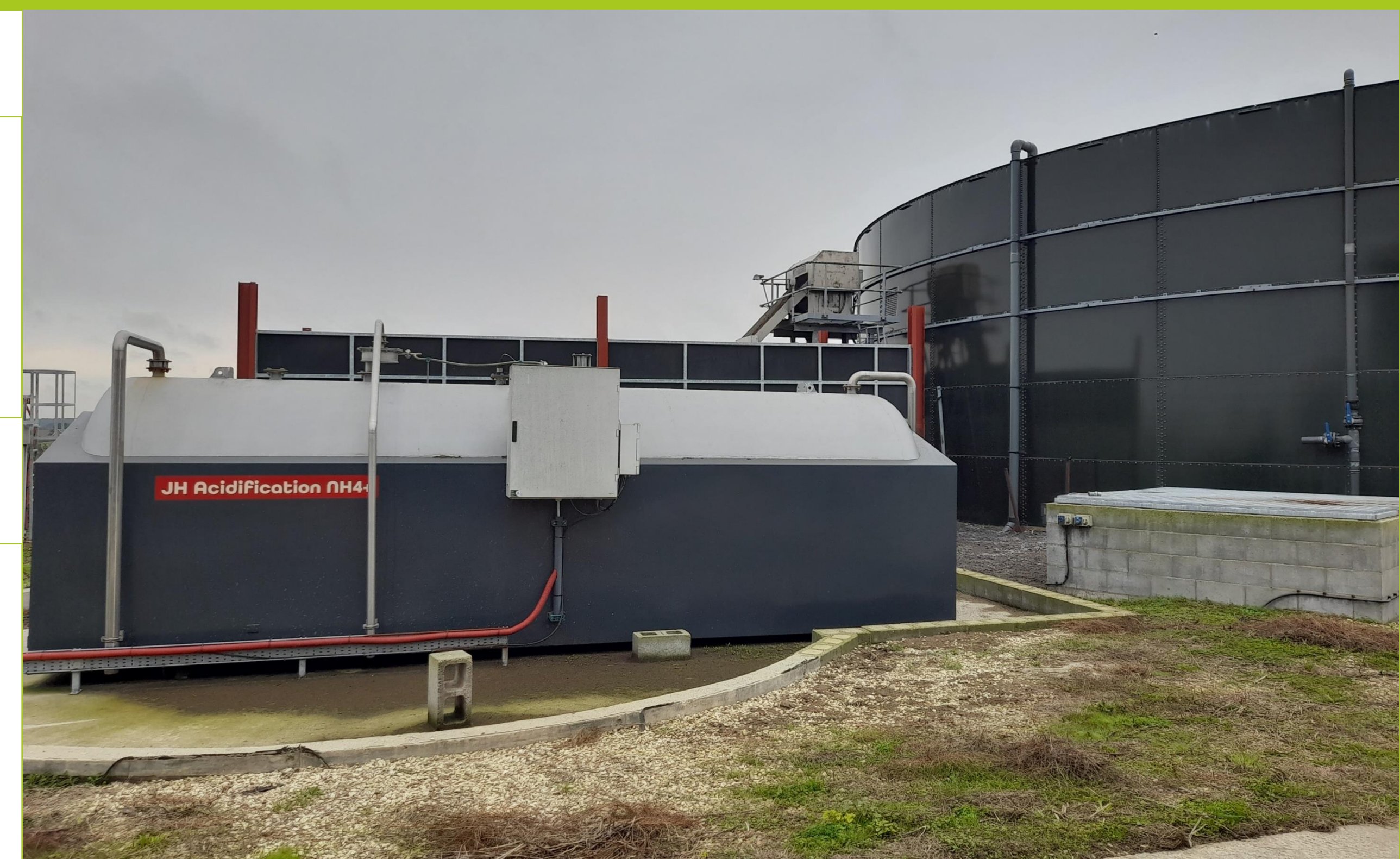
Image 1: In-house acidification system on a UK pig farm
