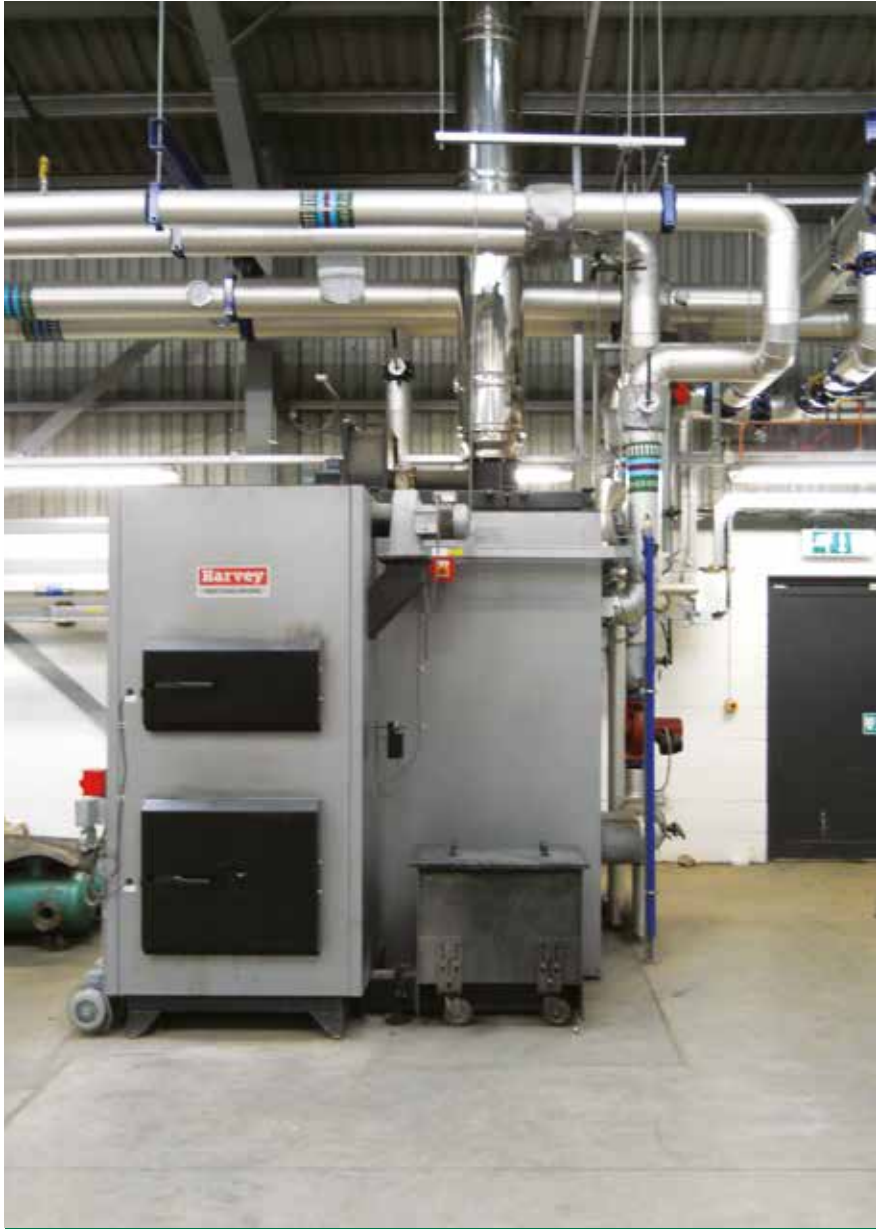
Froling (320kW) Biomass boiler utilising woodchip at AFBI Hillsborough
