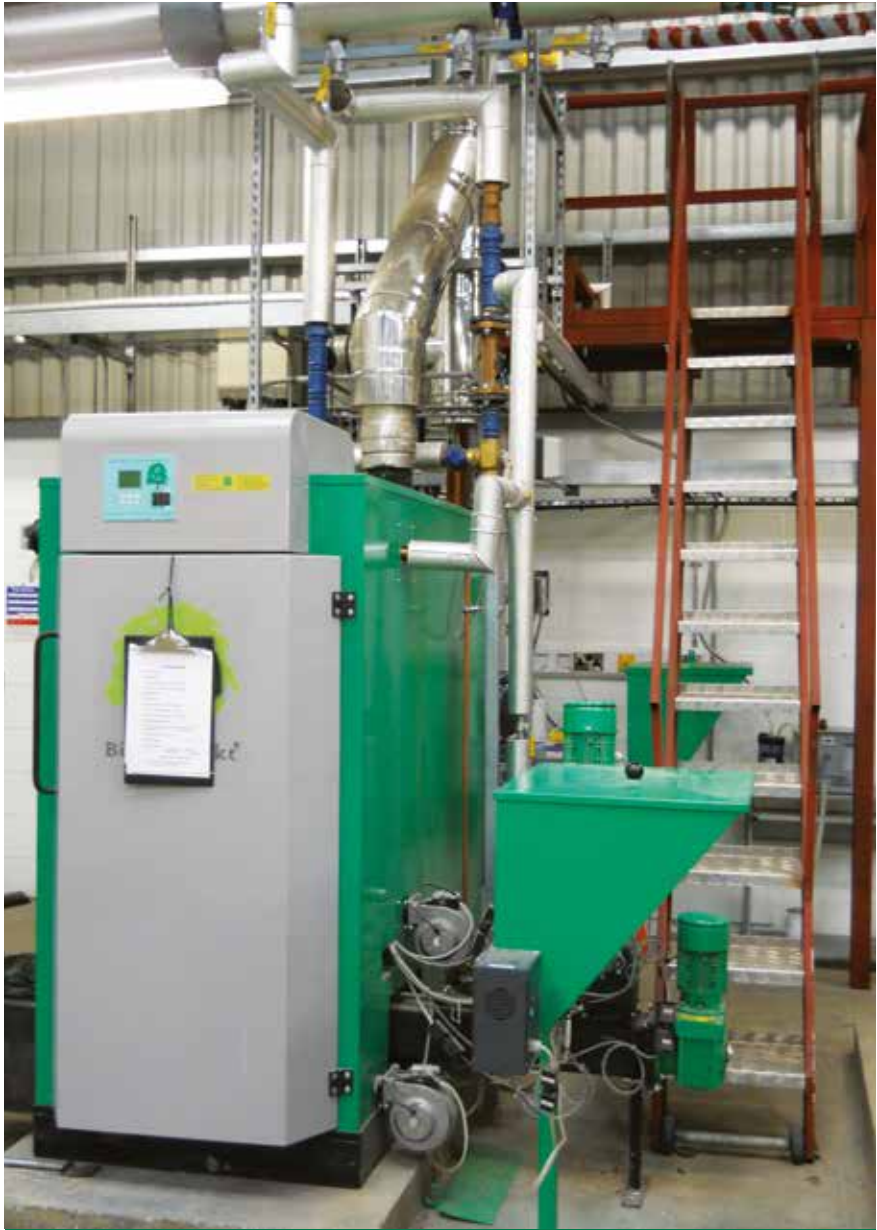
Biokompakt 120kW AFBI Hillsborough boiler system showing chip bunker external combustion
