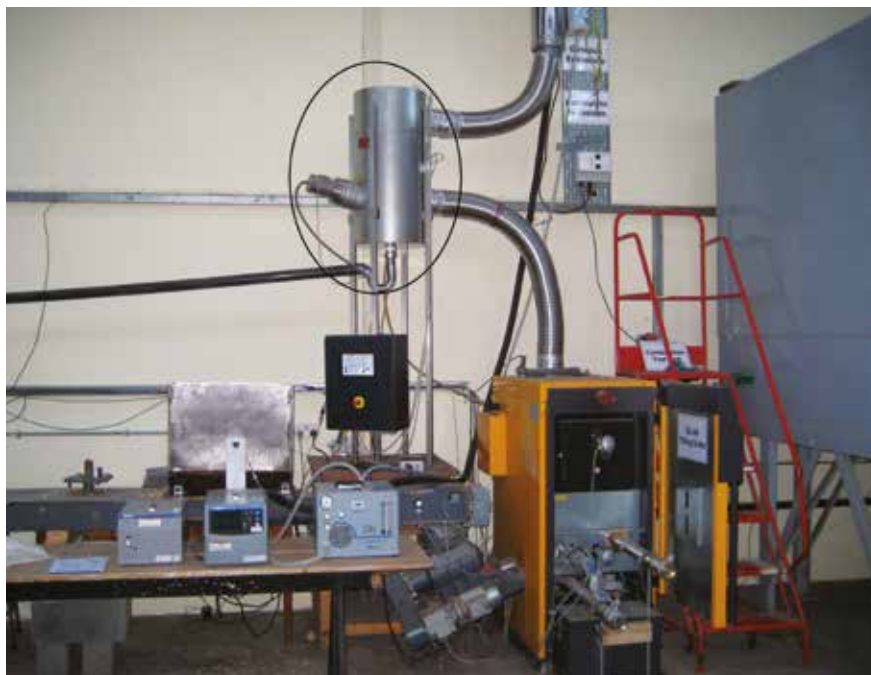
Combustion test bed at Teagasc, Oak Park fitted with electrostatic precipitator to reduce particle emissions during combustion
