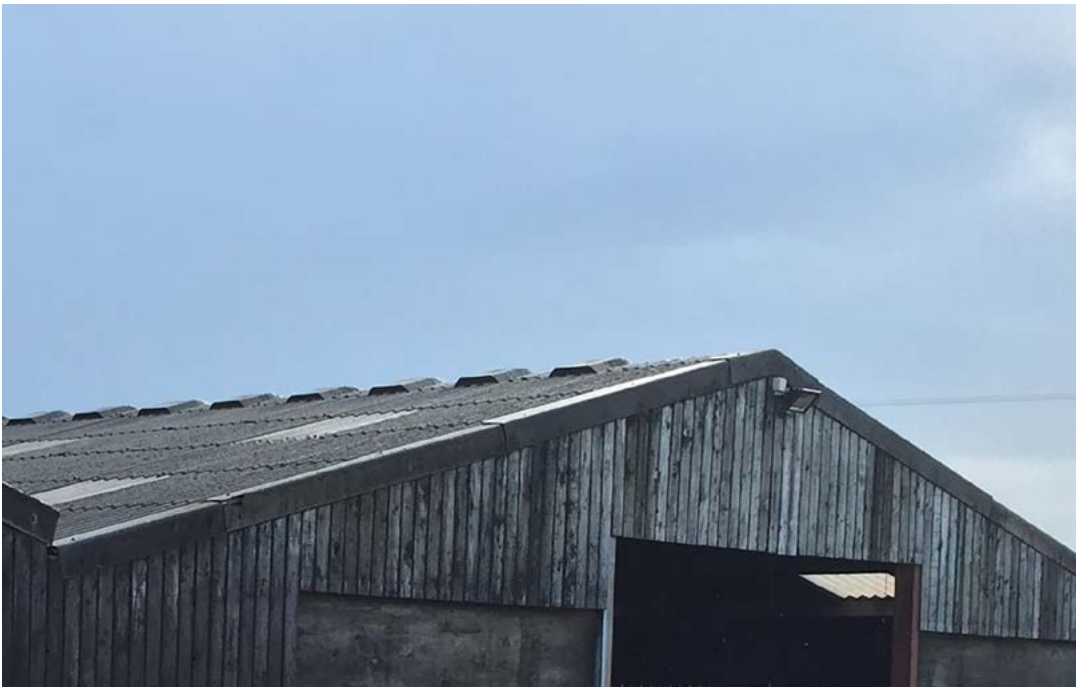
Ventilated ridge – inadequate. These ridges often supply less than 30% of the ventilation needs
